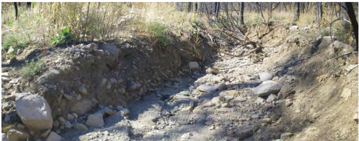
Figure 88. Representative photo (ID6) of the incised channels found in the less steep reaches of the upper Siesta-Paintbrush watershed
