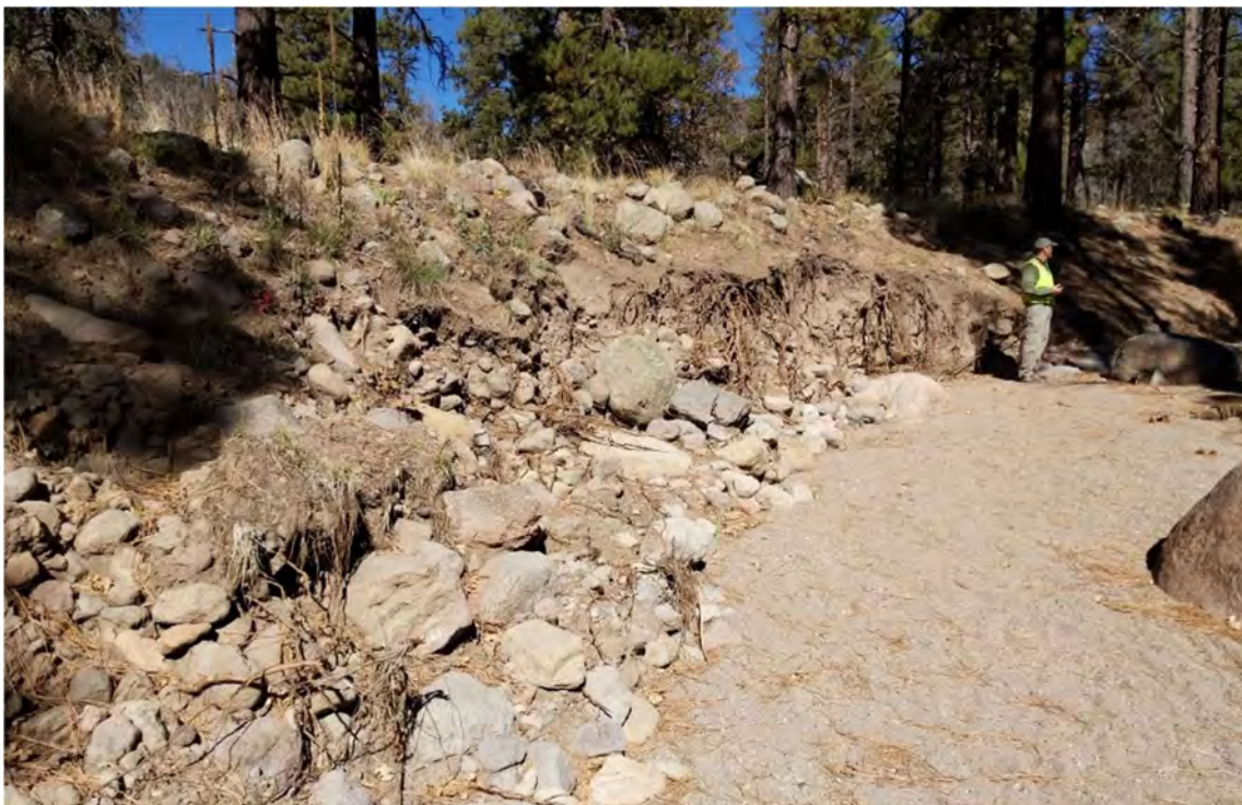
Figure 4. NCD surveyors completing the BEHI analysis on a typical channel along Spruce Ave Wash.
