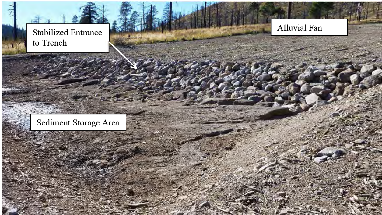
Figure 16. Trench in a fan in the Schultz Fire area.
