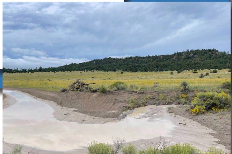
Looking downstream from plugged headcut to leadout channel. (Photo courtesy of Keystone Restoration Ecology)
